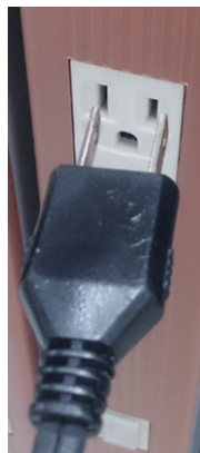
Figure3. Power outlet connection
